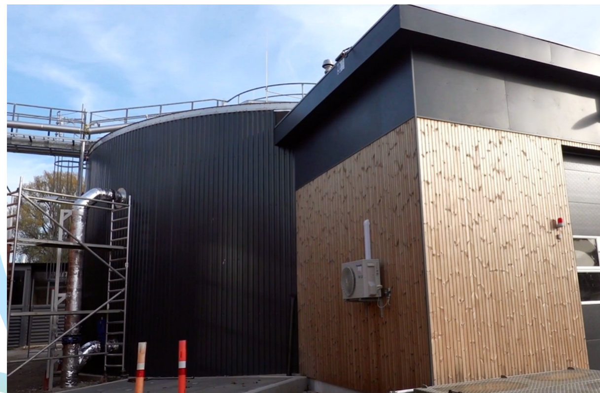
Steel Sludge Storage Tank - VCS Denmark
